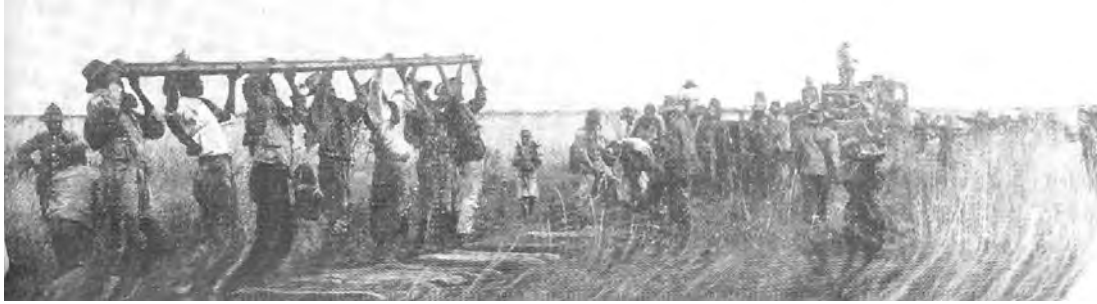
A photograph showing the construction of the Otavi Railway across Herero land in 1903.
